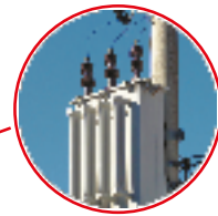
outdoor and overhead switchgear
