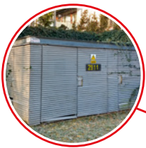
outdoor and overhead switchgears
