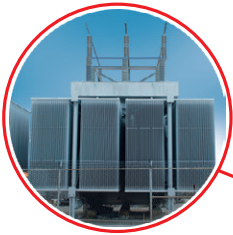
HV/MV transformer bay
