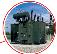
HV choke bay
